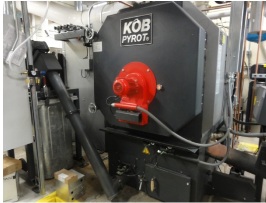
Ash -Boiler-Fuel Feed
