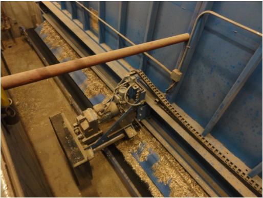
Automated Fuel Handling
