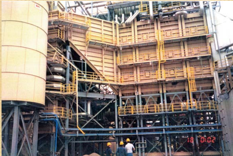
Energy and Heat 25 MWe FB Combustor and Boiler (EPI)
